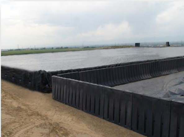
Primary & Secondary Containment
